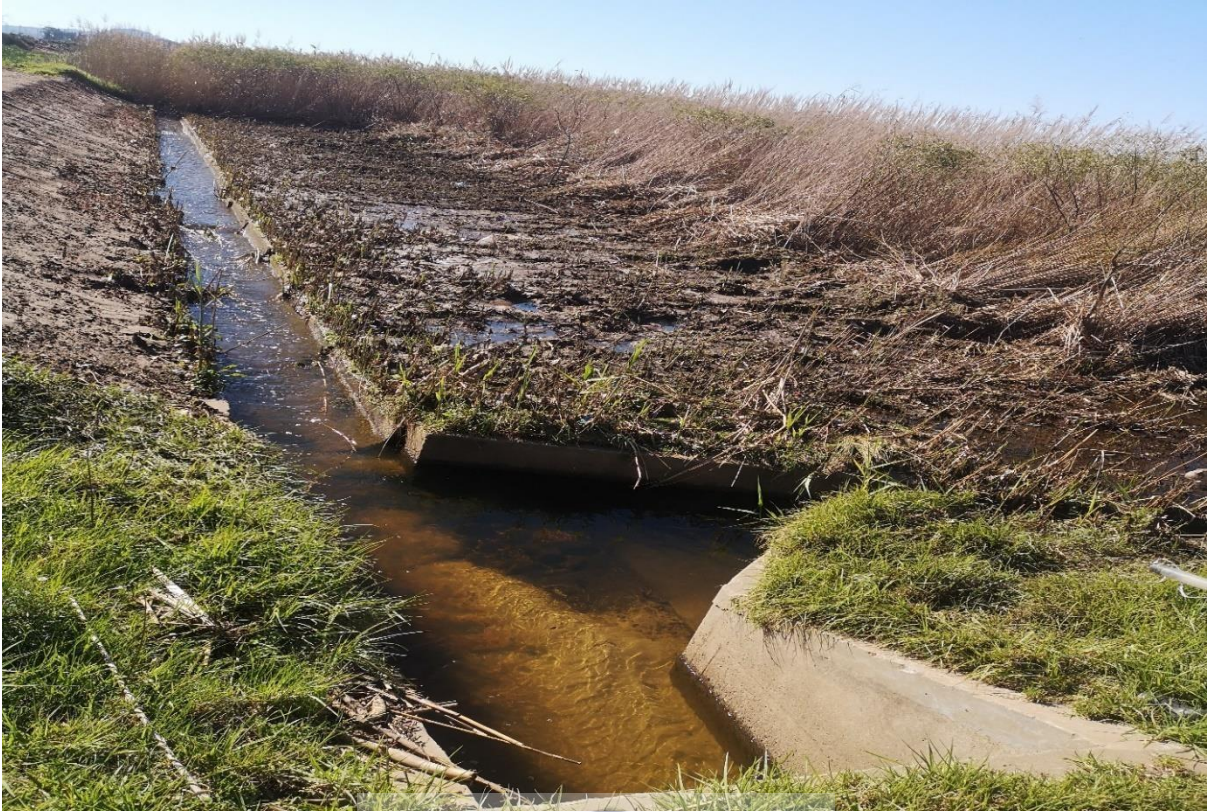
Figure 7: Atlantis water system basin 6 meeting with a combination of Basin 7 and 12.
