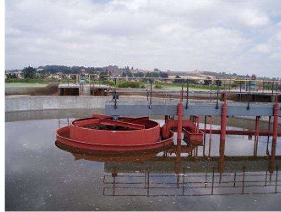
VI. Maturation pond (further purification of the relatively clean wastewater takes place)
