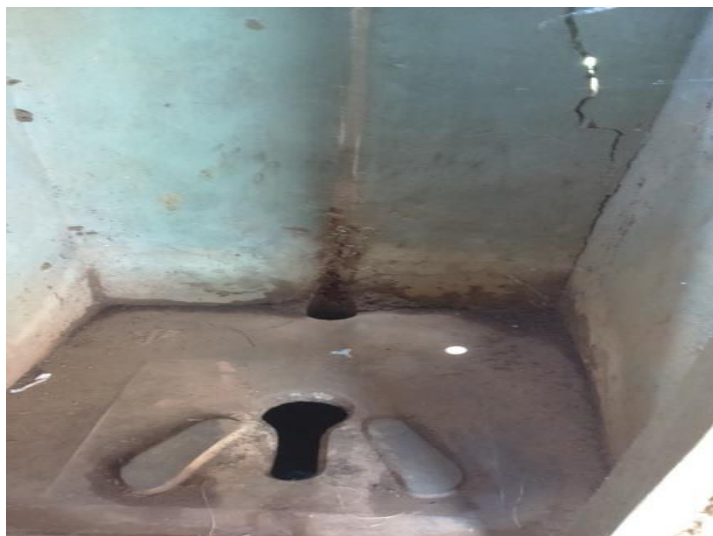
Figure 5: The only pit latrine at school for all learners
