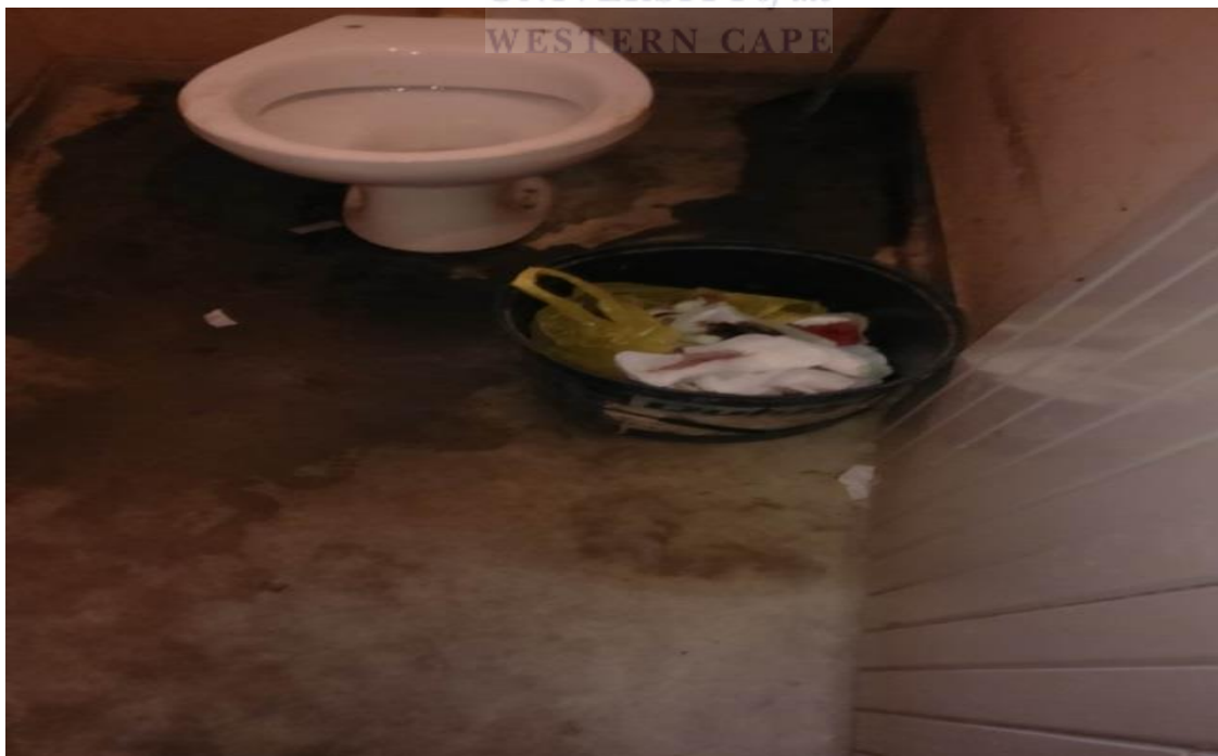
Figure 8: Toilet cubicle with sanitary pads in a flush toilet at school
