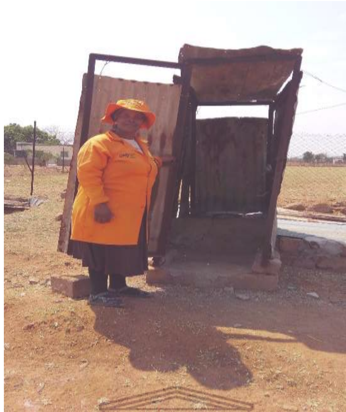
Figure 6.1: Dilapidated pit toilet without ventilation
