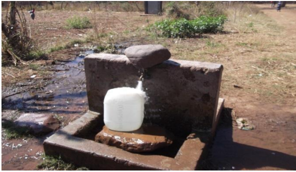
Public water point taps (community taps)
