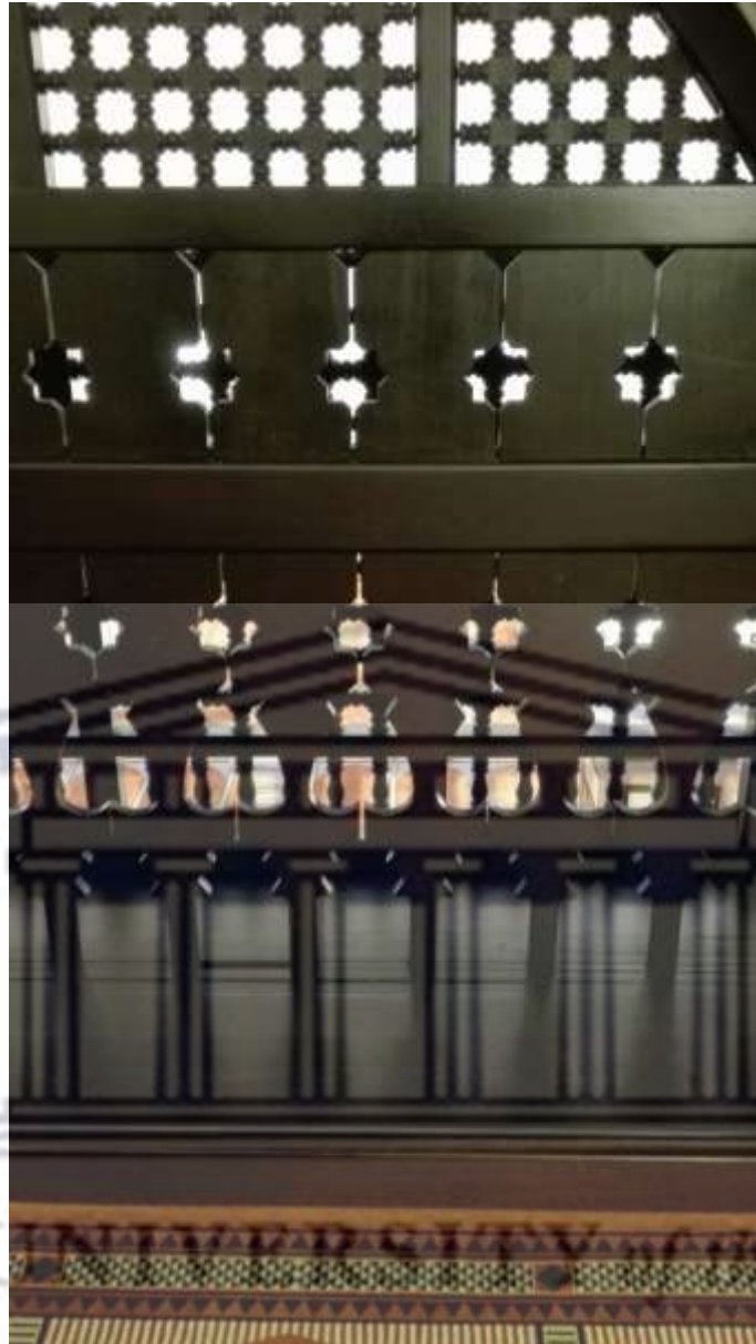
Figure 5. 47 Close-up of the decorative woodwork obscuring the view over the balcony and concealing the space from the men downstairs
