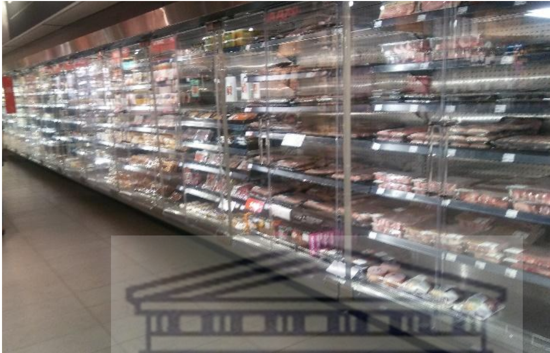
Figure 4.44: Woolworths A Fridge
