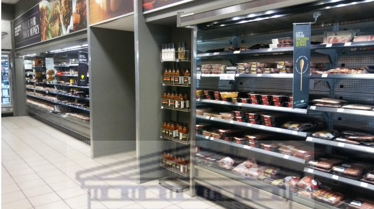
Figure 4.47: Woolworths C Shelved Fridge
