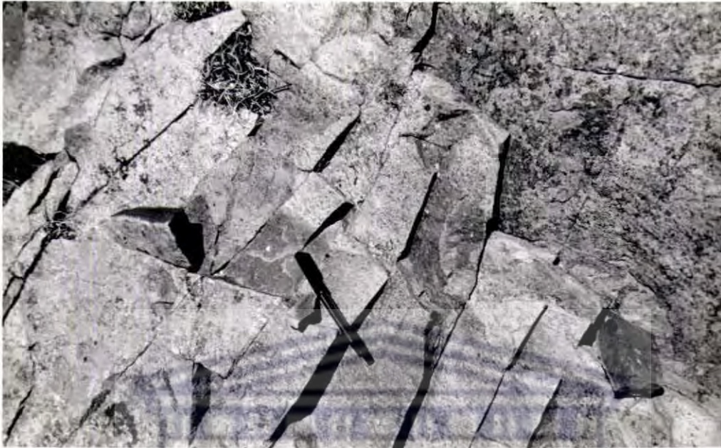
Figure 66. Cubic fracturing in clay-rich sandstone may be related to hydration of clays or volume changes upon chemical alterations.
