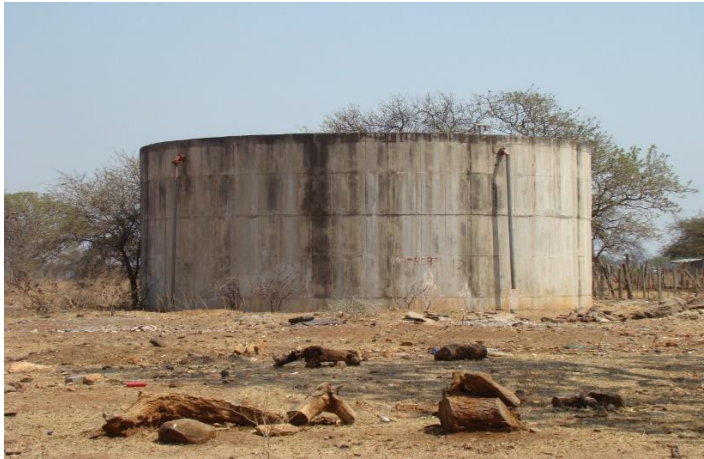
Figure 5. 14 Mayephu village reservoir about 1 km from borehole; cost of fuel to pump water into the reservoir is very high.
