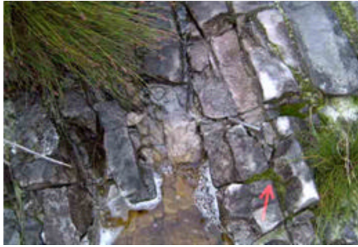
Figure 6.5 Fractures clogged with infillings near the surface in the Table Mountain
