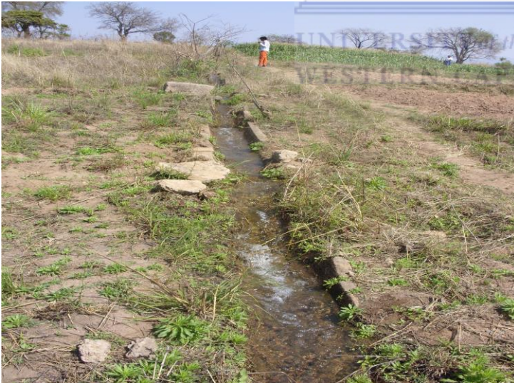
Figure 10: One of the broken canals channeling water to the farmers' fields
