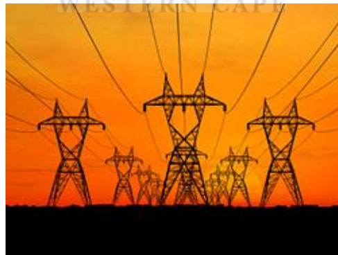
Figure 2.1: Power lines that transmit electricity
