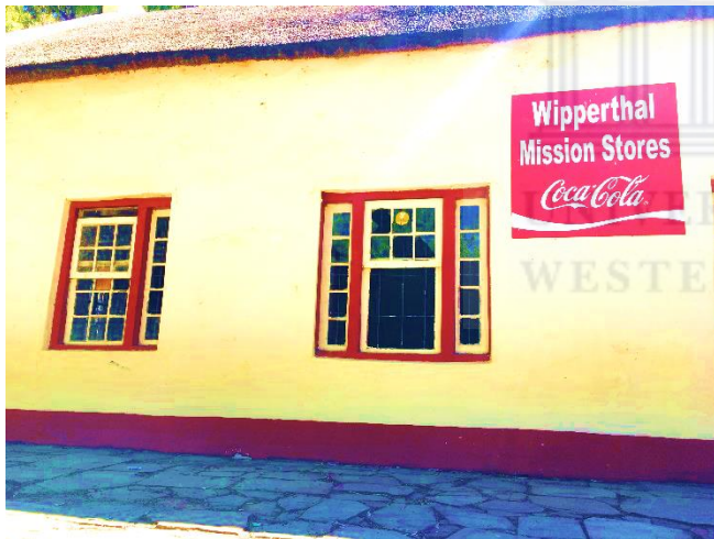
Figure 19: Neglected Mission Store with broken windows
