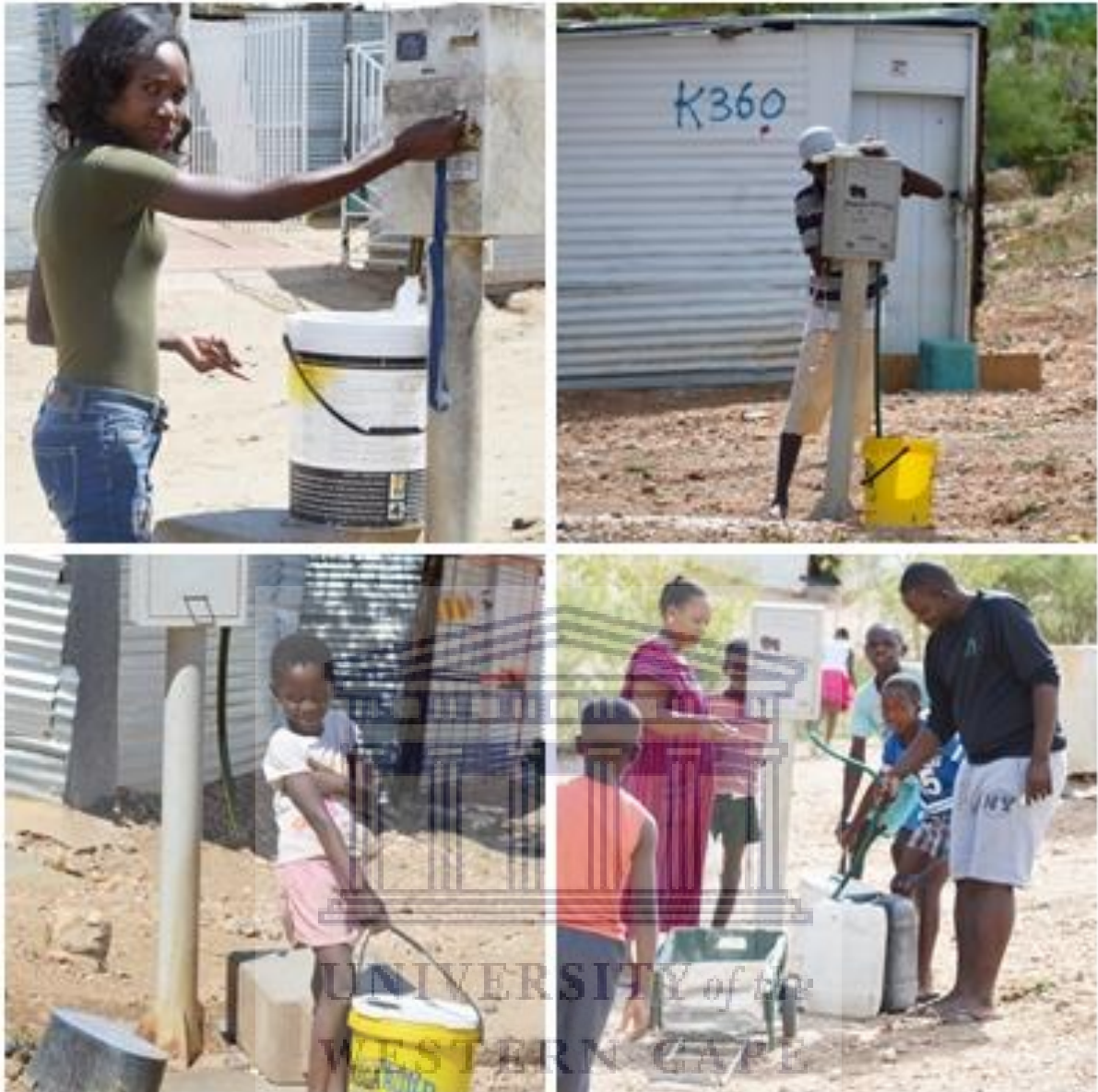
Figure 5.6: A photo of the Water tokens and water-vending machines taken by the author in Havana informal urban settlements, Windhoek. December 11, 2017
