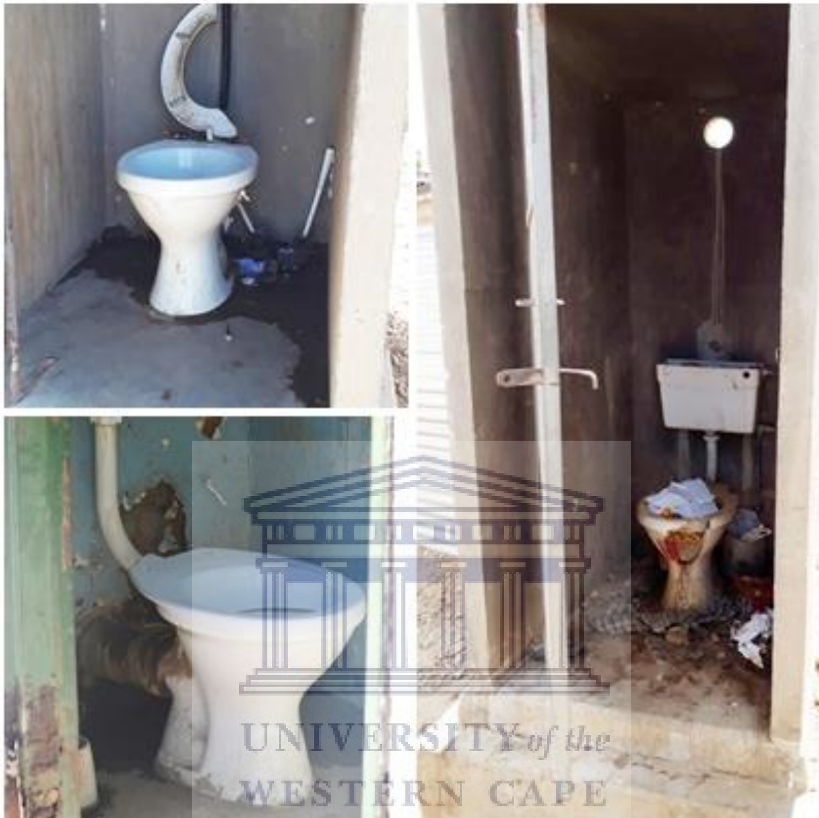
Figure 5.10: A photo of the Communal toilets in the Havana informal urban settlement taken by the author in Havana informal urban settlements, Windhoek. February 10, 2018
