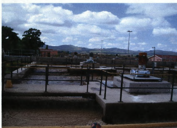
III. Aerobic pond (mechanical aerators introduce air to the wastewater)
