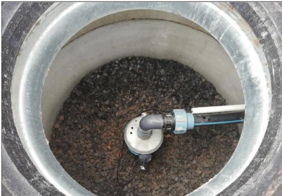
Figure 4.6: Boreholes equipped with injection pipework and submerged probes inside the borehole in one of the injection boreholes (10DNE) once the manhole casing was removed at the study site, Atlantis (Nhleko et al., 2020).
