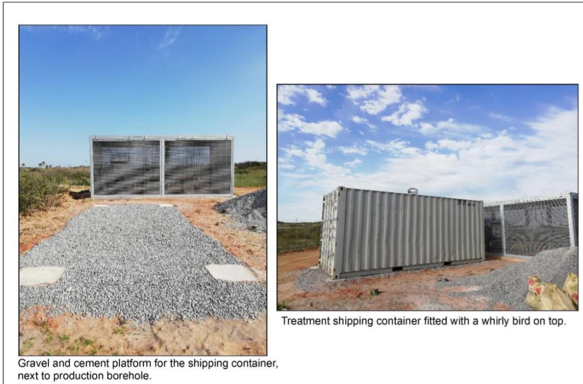
Figure 4.2: The shipping containers position and base design at the study site, used as the groundwater treatment plant, and the production borehole (G30966) enclosed in the perpendicular cage (Nhleko et al., 2020). The base design used gravel and cement for stability.
