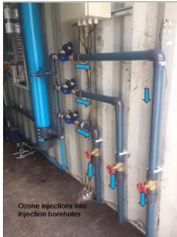
Figure 4.7: Ozone ( O_3 ) injection into injection boreholes after groundwater treatment using ozonation inside the shipping container at the study site, and the flow direction from the container into injection boreholes. Injection boreholes include 7DE, 11DNE, and 12DN.
