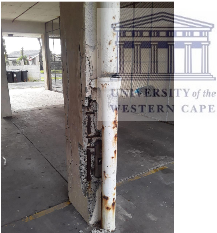
Figure 3: Gatesville damaged pipes (Community Leader, 2020)
