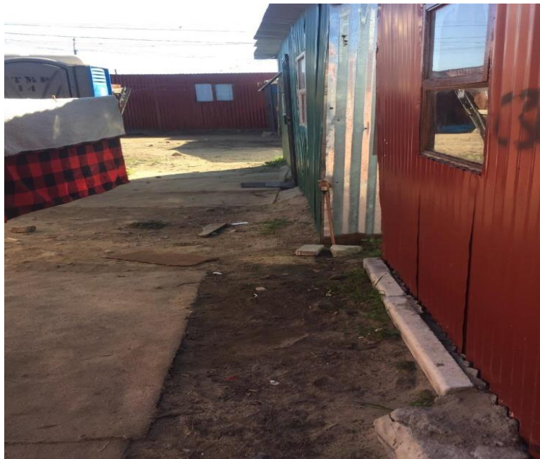
Figure 3: Water taps installed by the community
