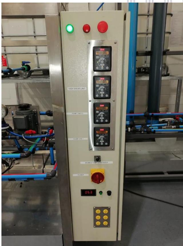
Figure 3.13. Photograph of the hybrid DAF shear unit control panel.
