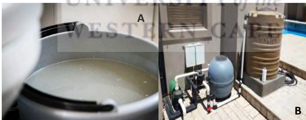
Figure 1.2: Examples of domestic greywater collection and storage. A: represents simple hand-bucket collection of shower water or washing machine run-off. B: Represents an intricate greywater collection and storage system attached to a home.
