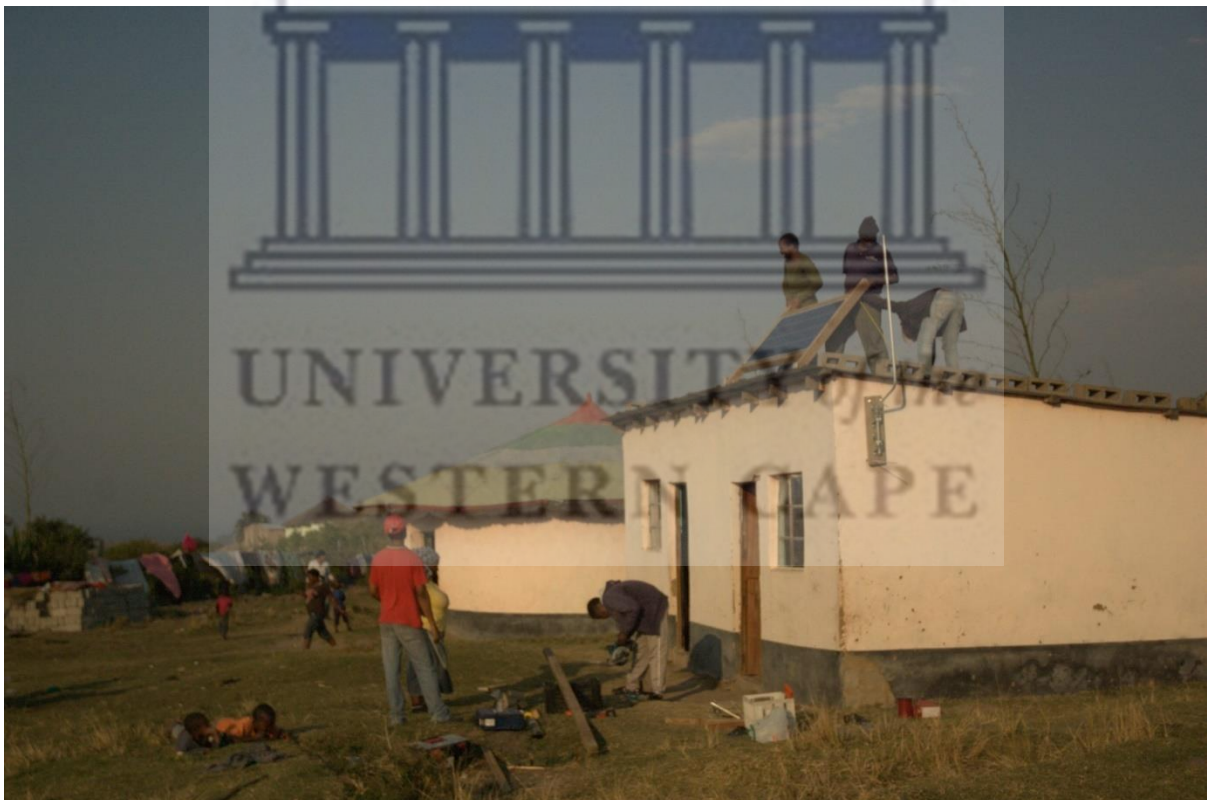
Figure 6: Mankosi resident installing solar system (DSI, 2022)
