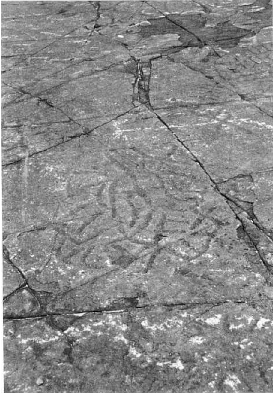
Plate 21. In October 2000 a front-end loader was used to scrape mud off the engravings on part of Driekopseiland, resulting in serious bruising of the surface (as seen in the foreground in this Plate), and further breakages in areas already subject to exfoliation (top of Plate 21). Fortunately only a relatively small portion of the site was damaged.
