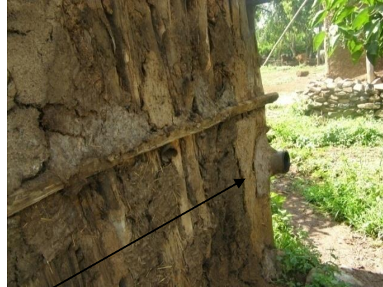
Fig 6: ventilation hole for removing smoke
