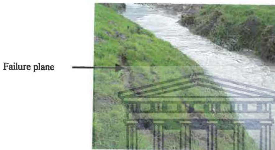
Plate 6.1: Failure plane along which the bank material on the right bank failed. The remaining material was still intact.
