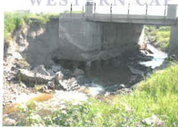
Plate 6.2: Undercutting of the Old Bottelary Road bridge pillars upstream of Site 1 – Photograph taken 02 September 2002.
