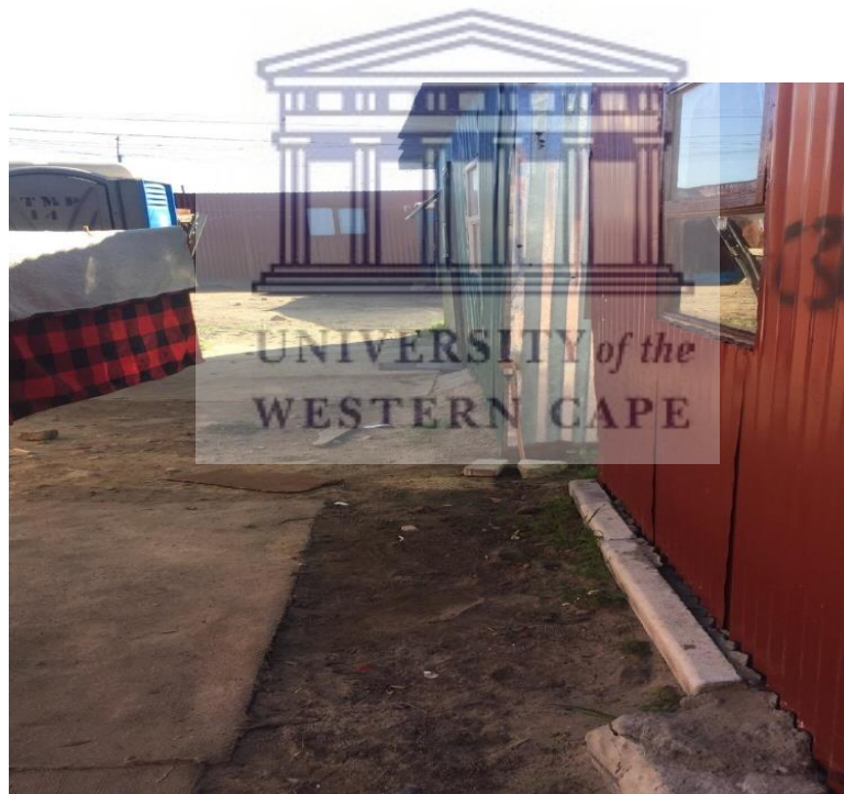
Figure 3: Water taps installed by the community
