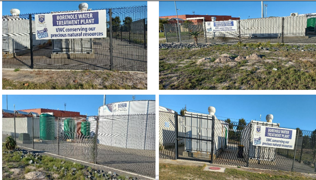
Figure 10: Photos of the Water treatment plant
