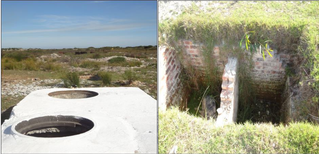
Figure 5.24: Open sewer and an open and damaged manhole
