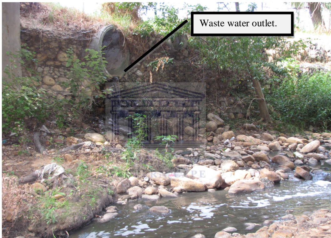
Figure 2.5 Municipal Treated Effluent Outlet located at FR7.
