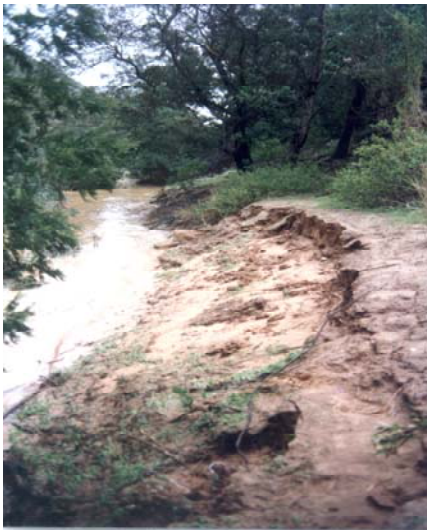
Plate 6.1 Erosion during high flow
