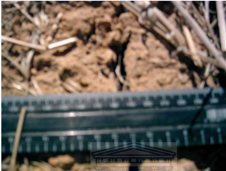
Figure 6.1 illustrating crack structure on the soil surface
