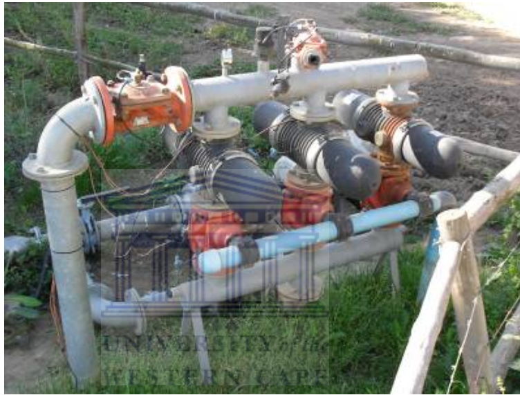
Fig. 7.2 Existing disc filtration system on the farm.
