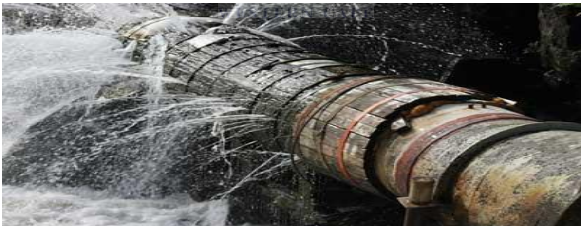
Figure 5: Broken water pipe
