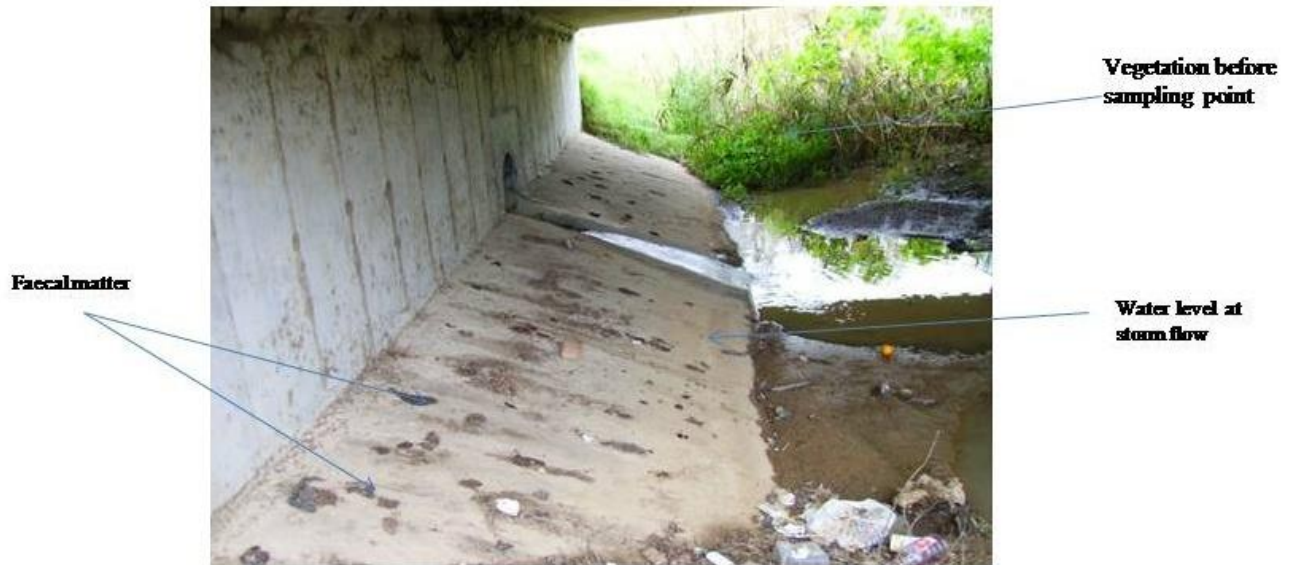
Figure 3.9: Conditions under the bridge at Pre-Khayamnandi at base flow after a heavy rain showing faecal deposits and vegetation in the river way.
