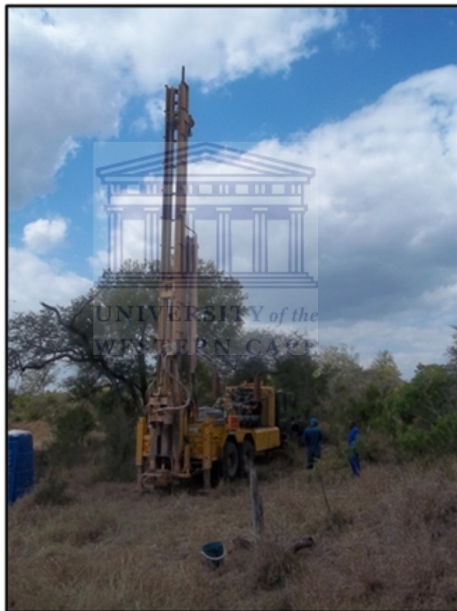
Figure 4.2 Super rock 5000 air percussion rig on a 10 ton 6x6 truck with 24 bar 900CFM compressor used for drilling the southern granite supersite boreholes.
