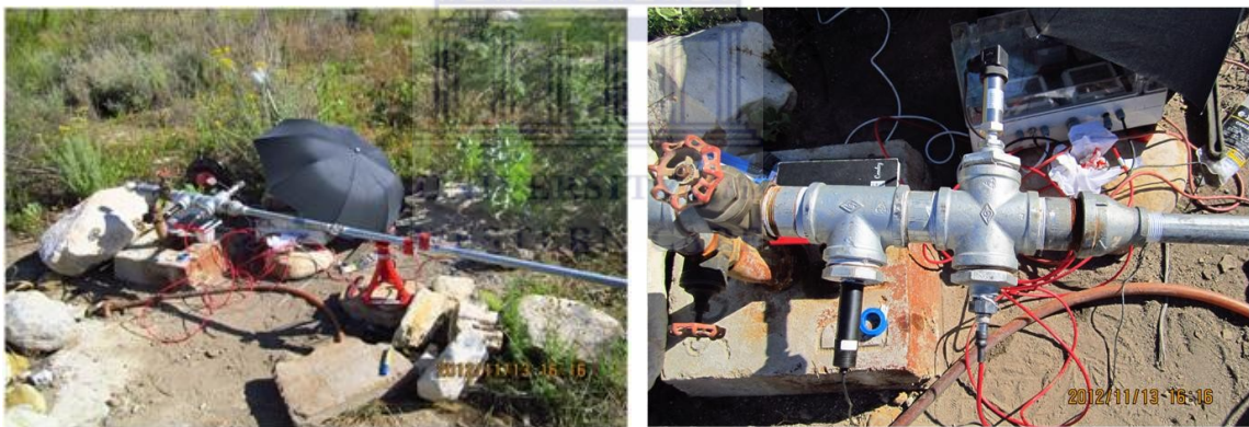
Fig. 4.12: The set-up of equipment test for measuring the flow rate and pressure of artesian borehole in Rawsonville
