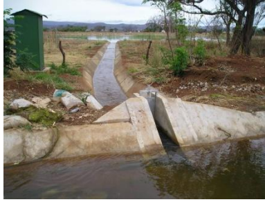
FIGURE 15 HEREFORD IRRIGATION SCHEME: WATER STORAGE DAM AND ABSTRACTION POINT ALONG LINED PORTION OF HEREFORD CANAL, 2004
