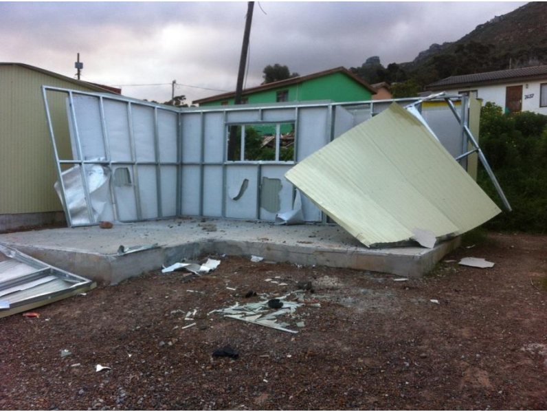
Figure 13, 14 and 15 show the vandalised temporary shacks. Photos taken by Roslyn Bristow, 2014.
