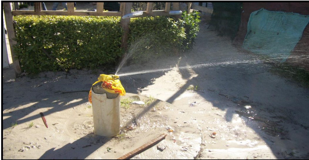
Figure 32: Broken Water Infrastructure in Nkanini Source: Sibanda (2014)
