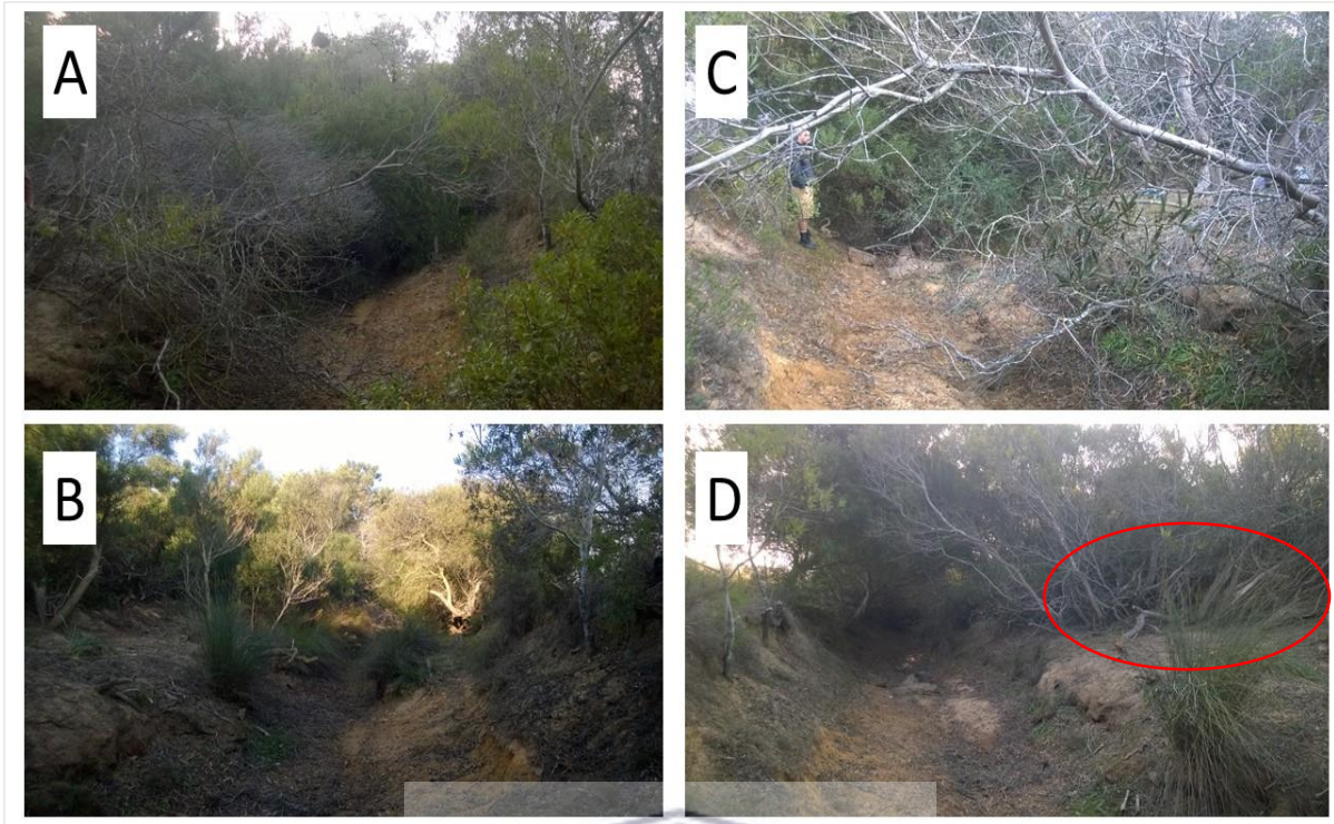
Figure 4.17: Downstream of the Elim Waste Water Treatment Plant flow monitoring site before and after clearing (A, B) and upstream of the site before and after clearing (C, D).
