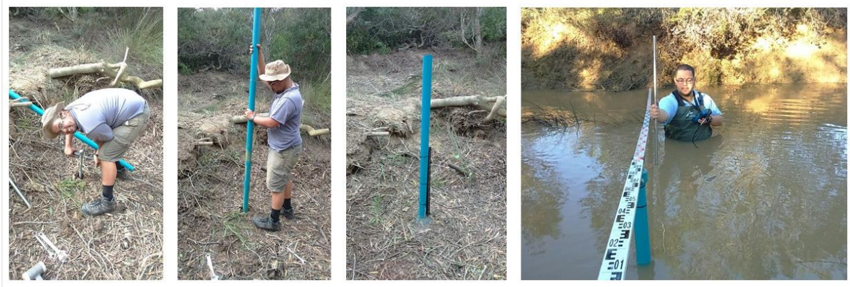
Figure 4.18: Installation of the stilling well and a flow measurement being done during one of the peak flows at Elim Water Treatment Plant.
