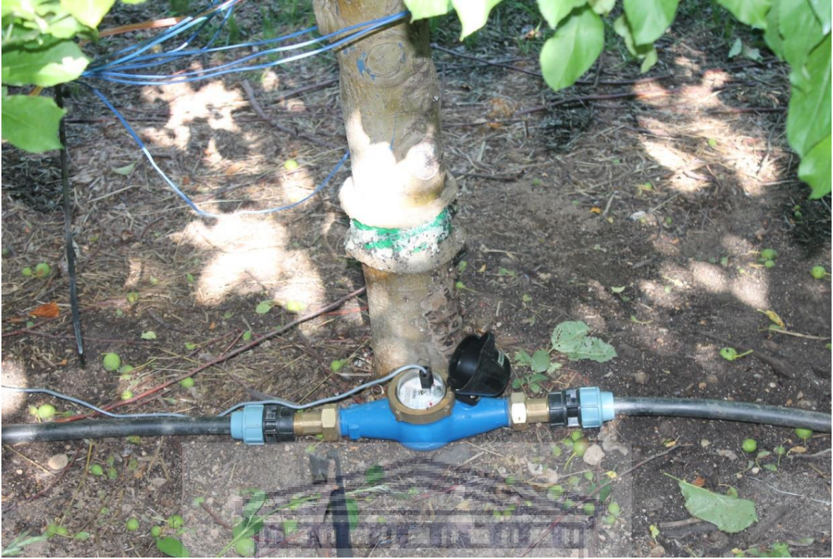
Fig. 4.3: Water flow meter measuring irrigation levels.
