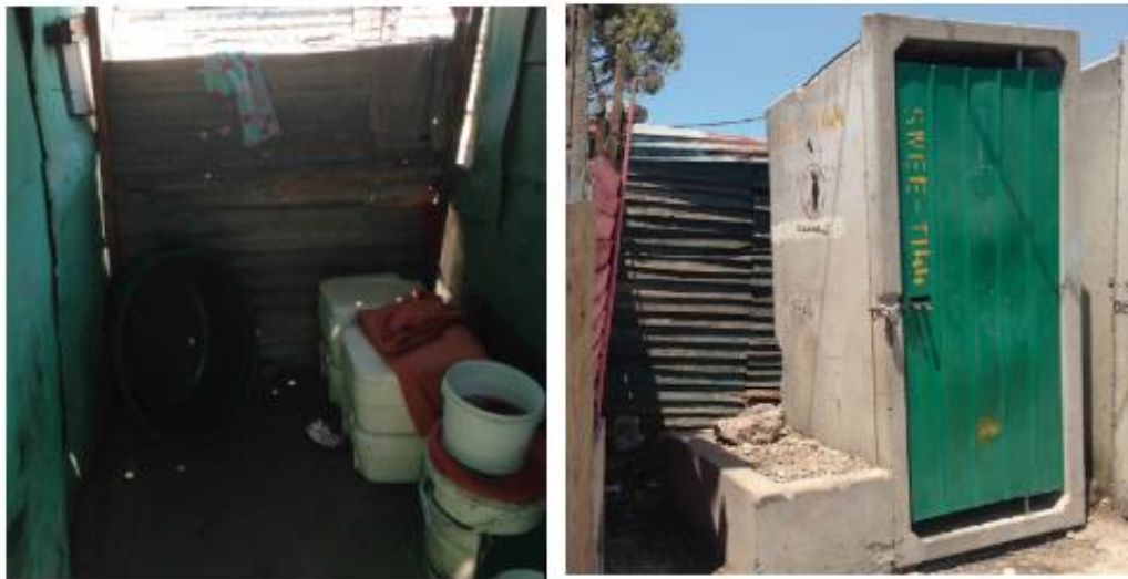
Figure 28 Anathi's portable toilet and the communal flush toilets available to her ECD in Sweet Home Farm
