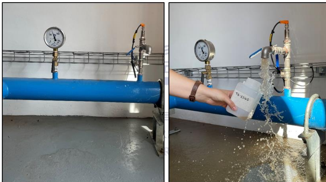
Figure 17: Sampling for major ions at production borehole HPF2-7 in the Hopefield Wellfield
